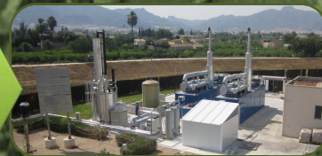
Biogas valorization: CHP
